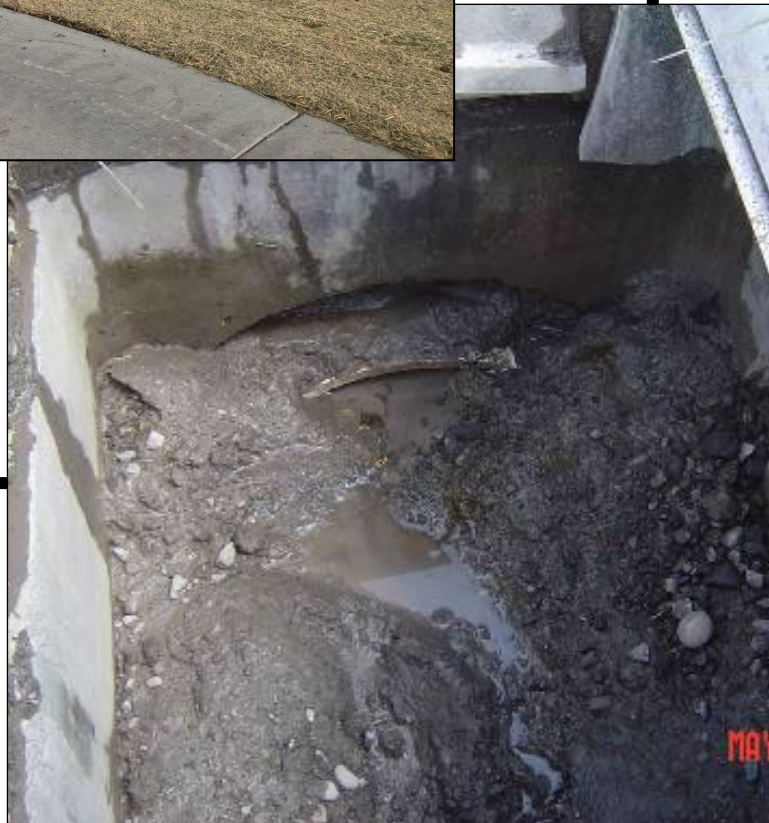
Graphic 5.0.2: Inlet sump clogged with construction debris
