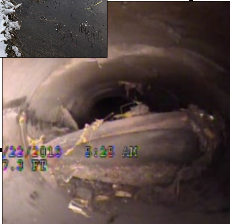
Graphic 1.0.2: Failed stormwater pipe
