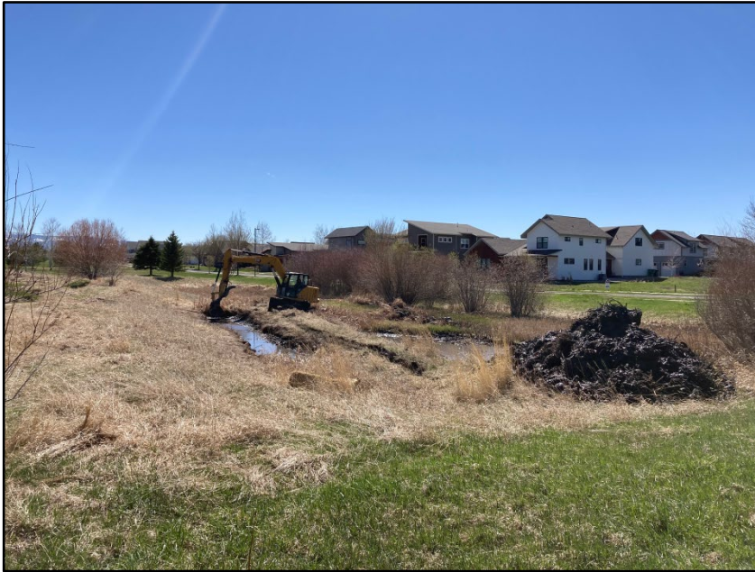
Graphic 6.0.1: Sediment filled stormwater basin during maintenance.
