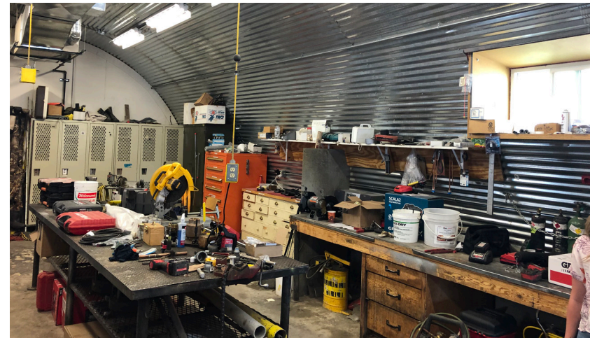
Existing Shop - Plumbing
